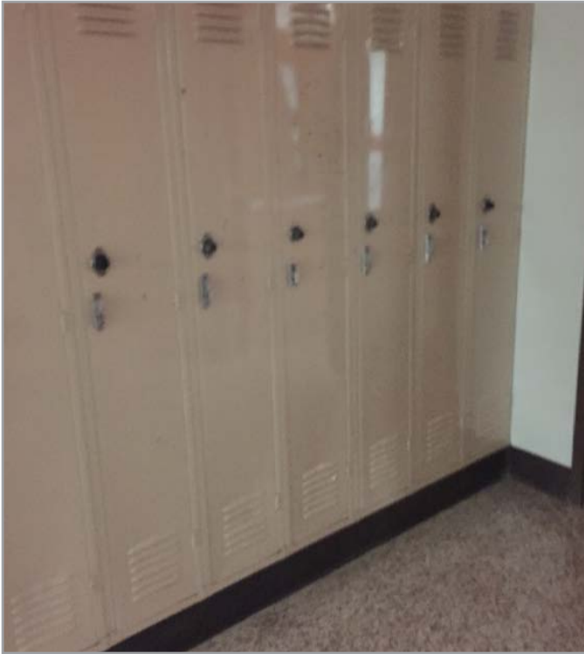
Damaged lockers in Corridor C162
