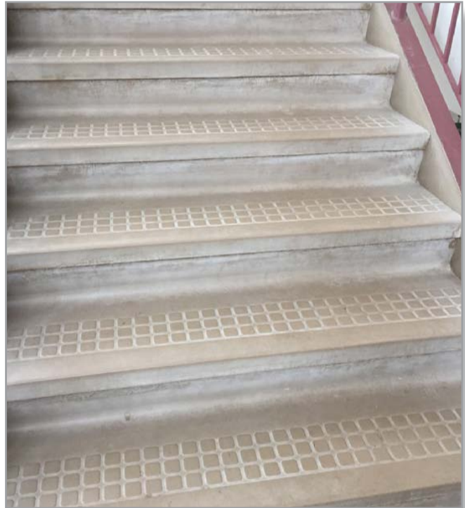
Faded stairway treads and risers needing replacing
