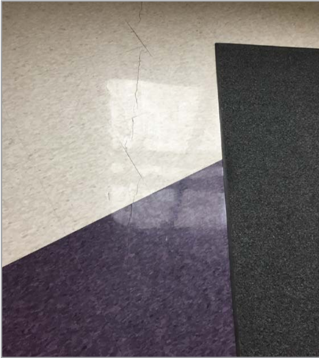
Damaged tile in Entry
