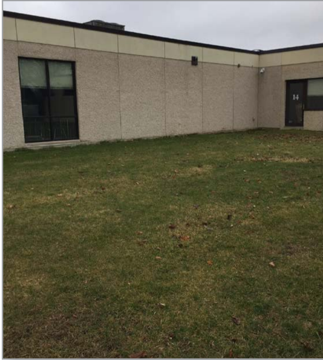
Soiled EIFS from roof
