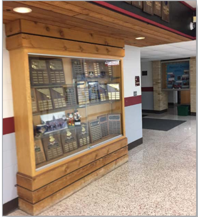
Display chase needs updating in Commons D100
