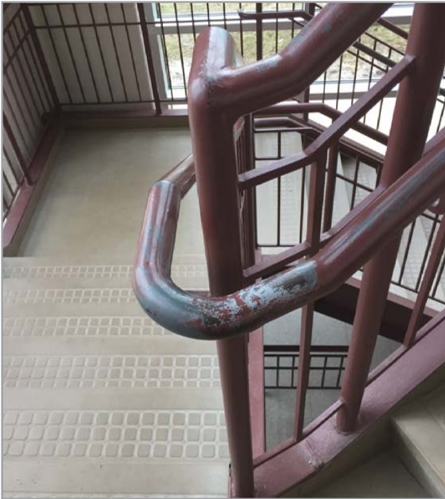
Stairway railings needing repainting
