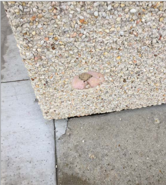
Damaged EIFS on exterior walls
