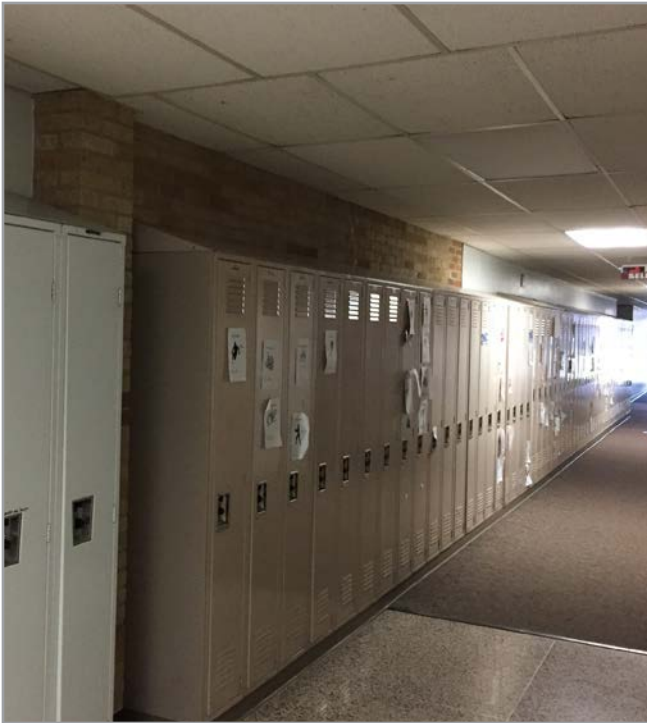
Corridor lockers in need of replacing in Corridor A149
