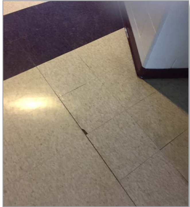
Damaged floor tile in Corridor
