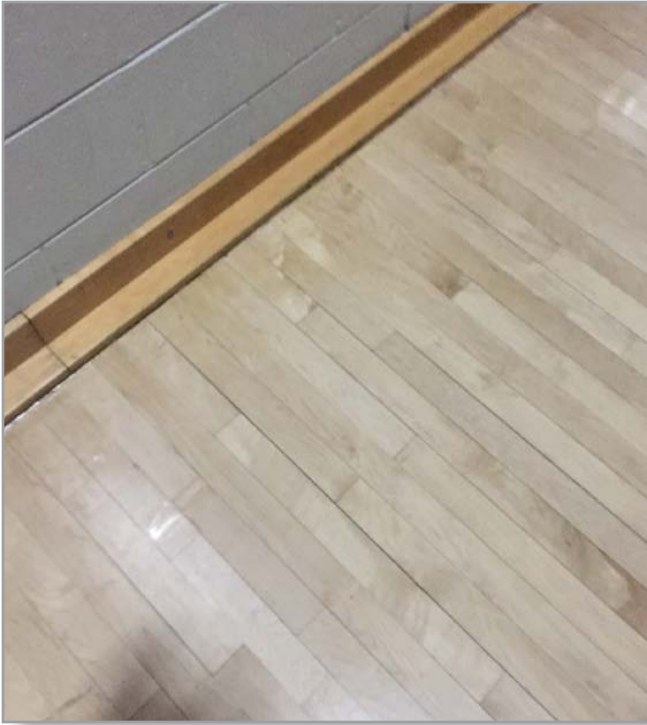
Loose gym floor base in need of replacing
