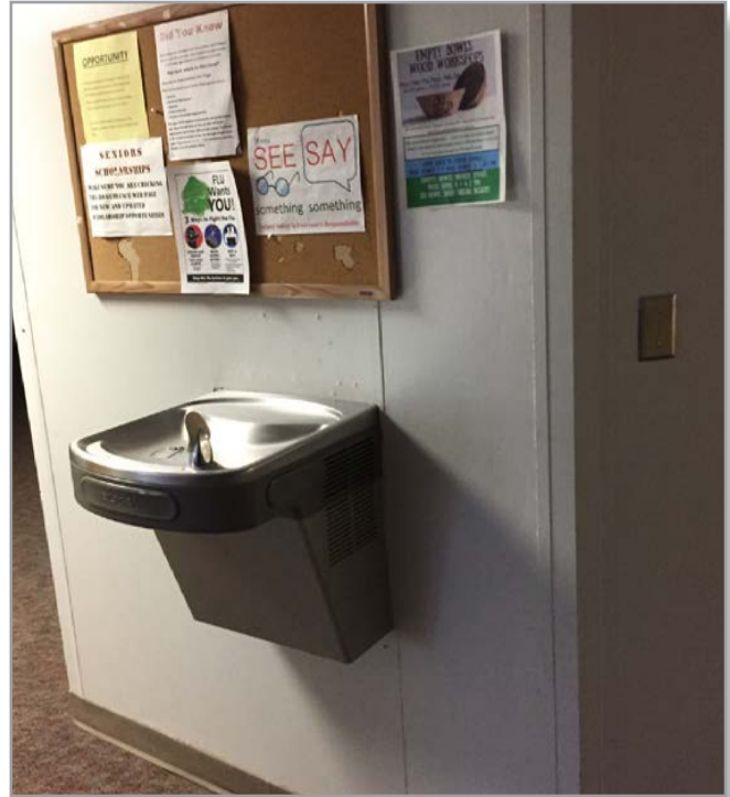
Provide high low drinking fountain in Corridor A109
