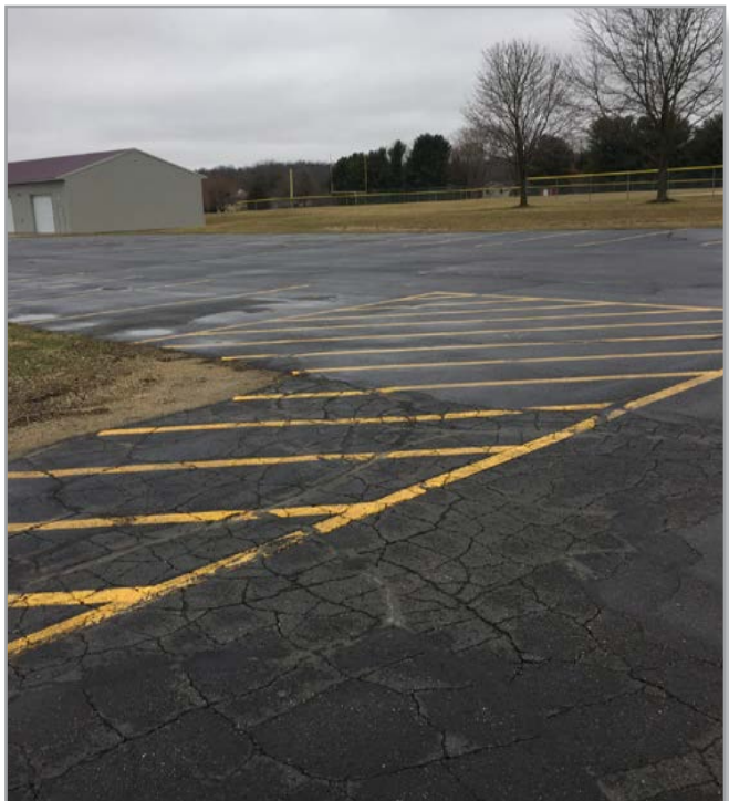
Replace damaged and worn asphalt
