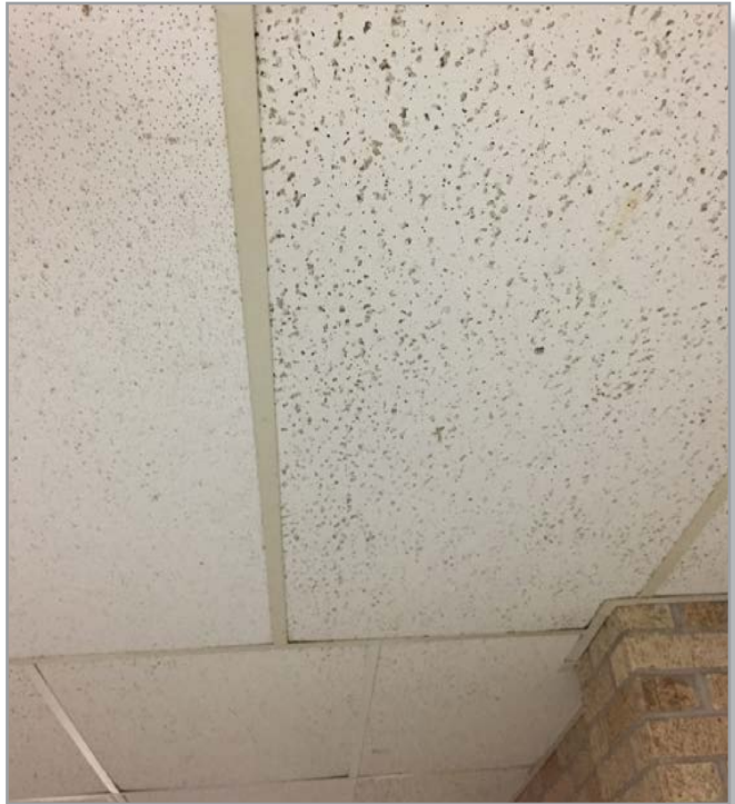
Different ceiling tile in Corridor A109
