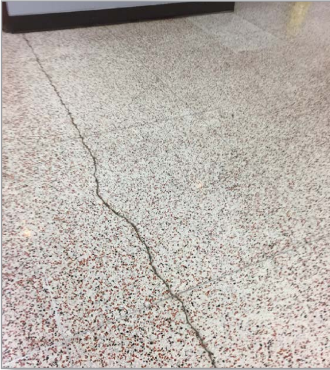
Terrazzo floor cracked in Lobby D101
