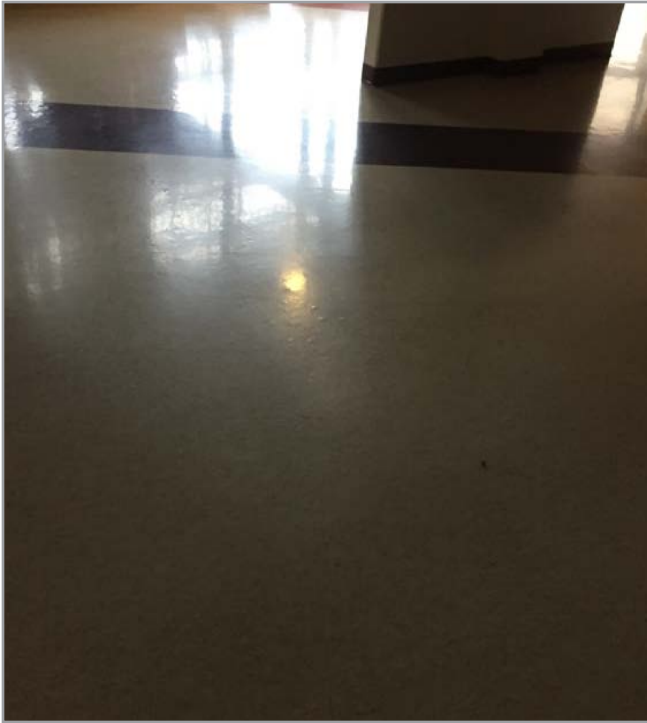
Cafeteria floor that needs to be replaced
