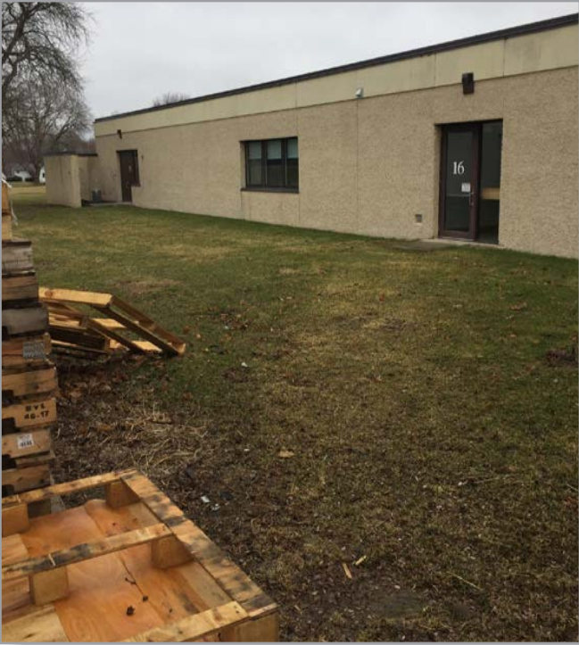
Exit door and frame in need of replacing
